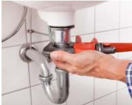
Check faucets, and pipes regularly for leaks and fix them immediately.
